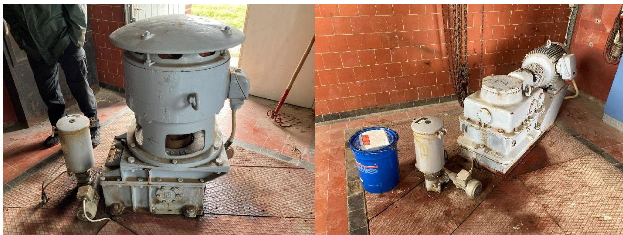
Figur 1.1: Pumperne i pumpestationen (26. august 2021).
